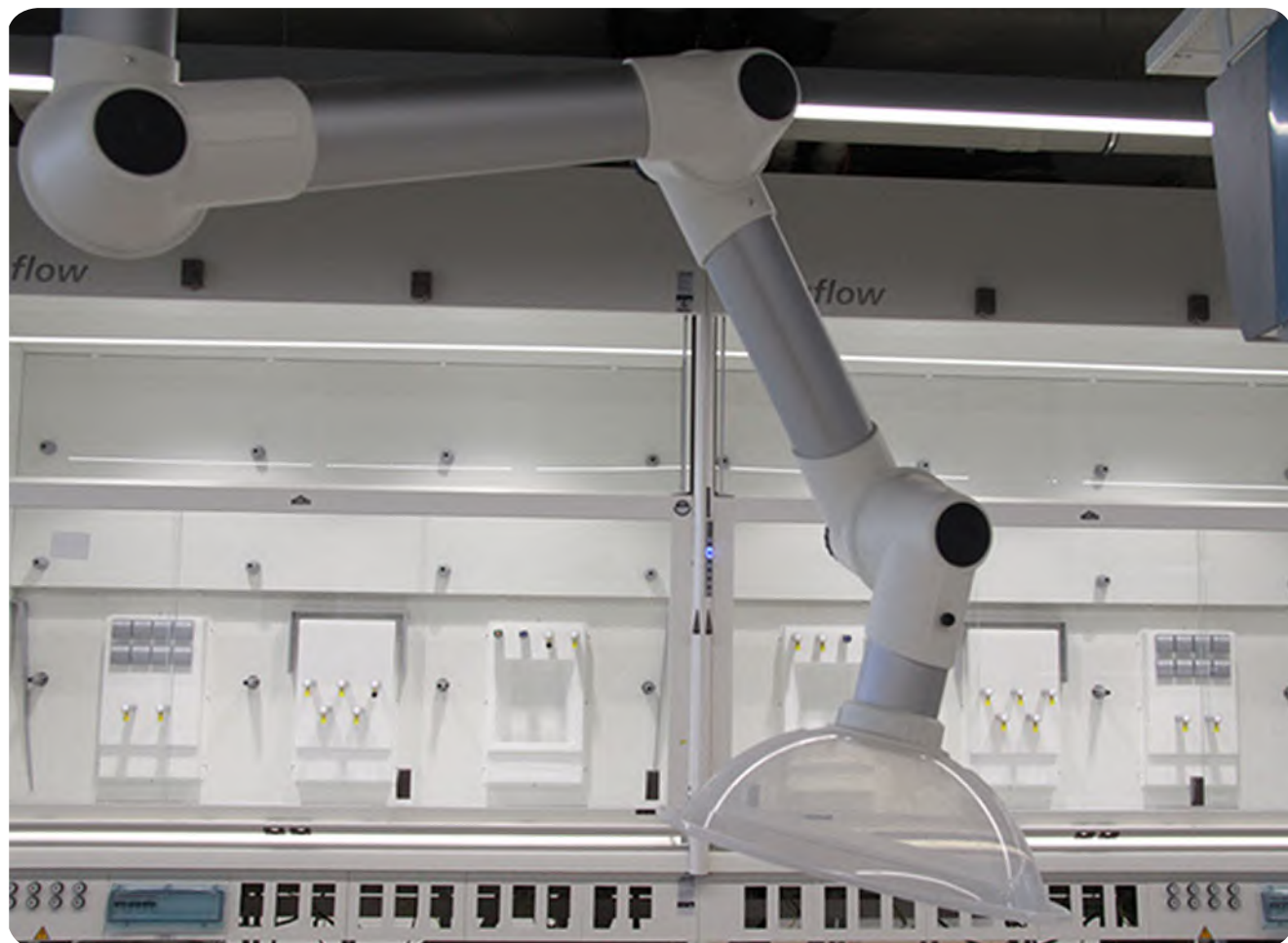
• Equipamiento del UPC Hydrogen Laboratory
